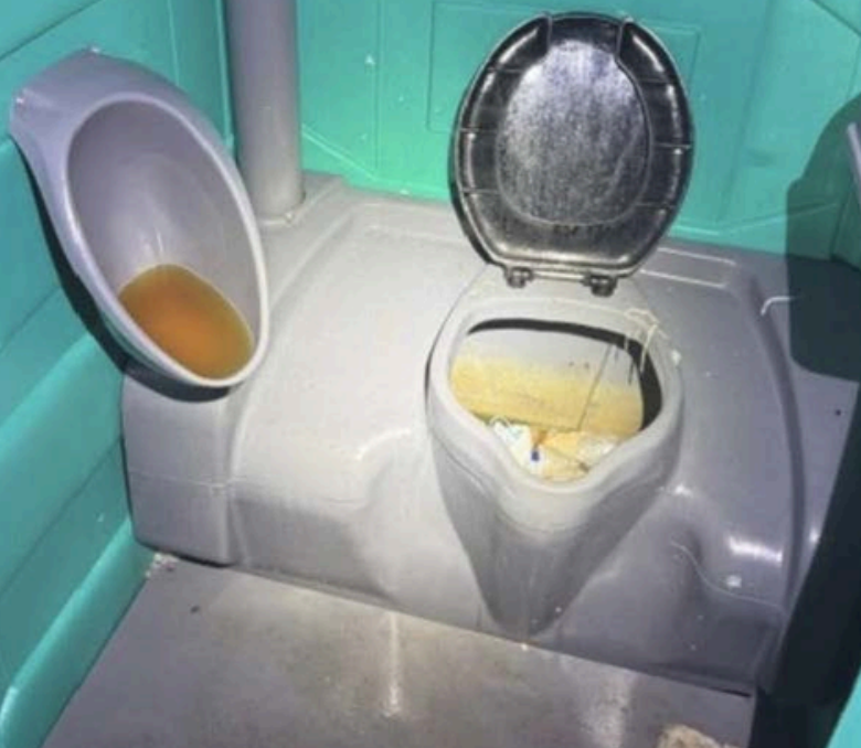
Inside view of one of the portable toilets located outside of the Miramar Holding Facility sally port. The portable toilets have not been serviced and are covered in human waste.
